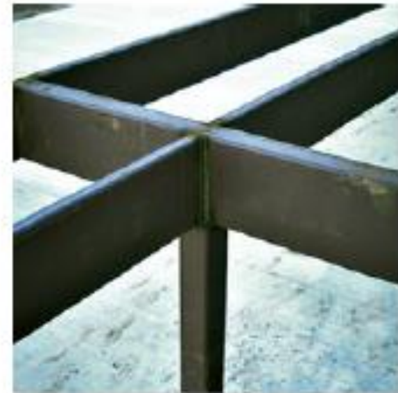
The floor beams of this building are welded together and thus form fixed connections. (10)
