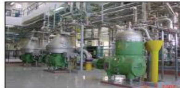
(i) Piping Network in an industrial facilities
